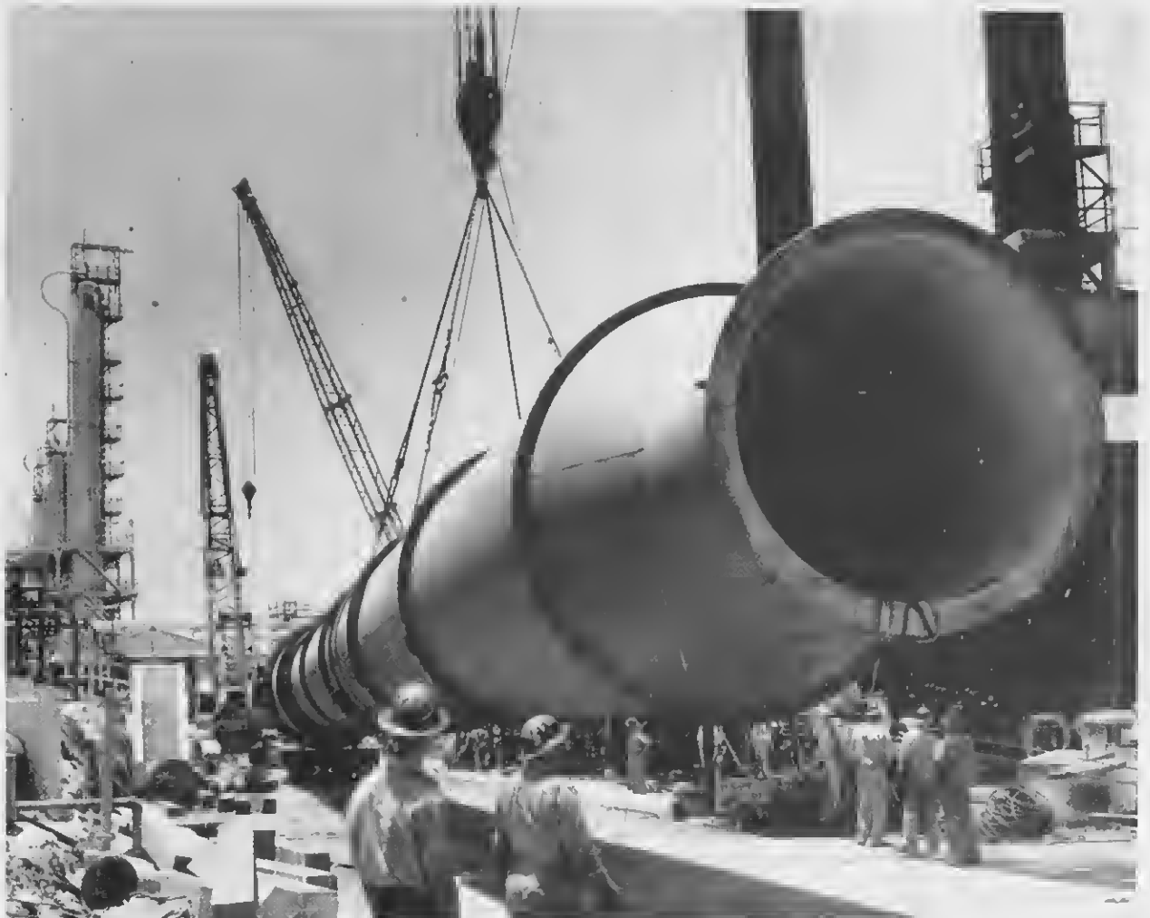
JUST BEFORE BIG LIFT, stack lies on side, lashings tight, load balanced, ready to be raised into place. POCO PROMER cu e trabao grandi a cuminsa, e staca ta na suelo, bon mara, balanza, cla pa worde hiza.
